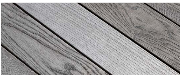
Unoiled Thermory Benchmark thermo-ash decking after 1 year
